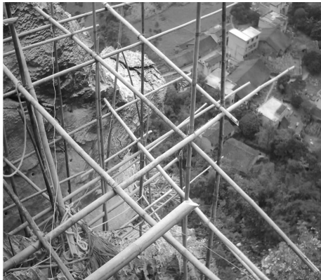
图 5 危岩与民宅的关系位置(在危岩上向南崖下拍照) Fig. 5 The relative position of the dangerous rock and the residential house(photographed from the cliff above the dangerous rock towards south)
