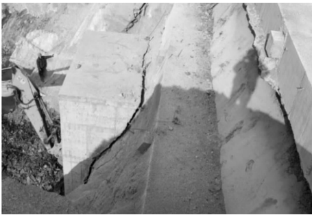
图 3 爆破后洞门混凝土开裂、分离情况 Fig. 3 Cracking and spalling of tunnel portal concrete after blasting
